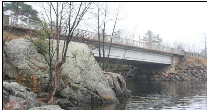
Figure 39 South Channel bridge showing bedrock of original shoreline on left and filled shore on right.
