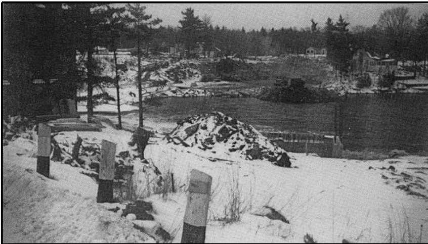
Figure 38 South Channel Bridge under construction showing land filling of bay. The old Presbyterian Church is in the trees on left. Source: Petry, Bala
