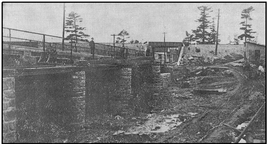
Figure 32 1913 bridge and dam under construction. The house visible through the railway underpass can be seen in Figure 20 Source: Petry, Bala
