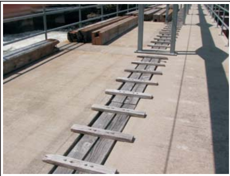
DAM DECK WITH UNSECURED STOPLOG GAIN COVERS
