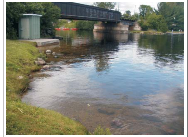
RAIL BRIDGE AT UPSTREAM END OF NORTH CHANNEL, NORTH ANCHOR OF SAFETY BOOM IN BACKGROUND
