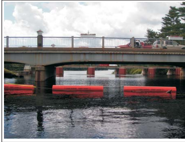
FROM UPSTREAM, DAM SHOWING OBSCURED DANGER SIGN
